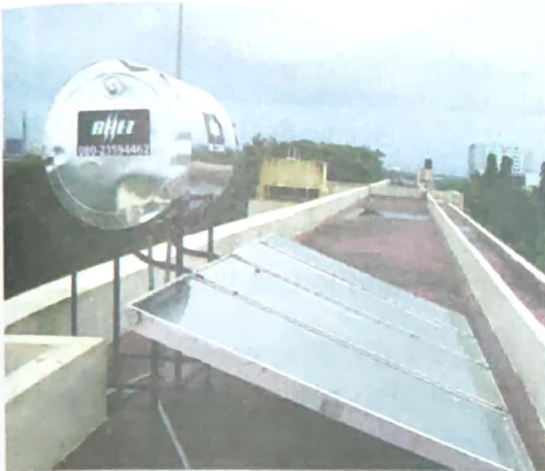
Solar water heater
